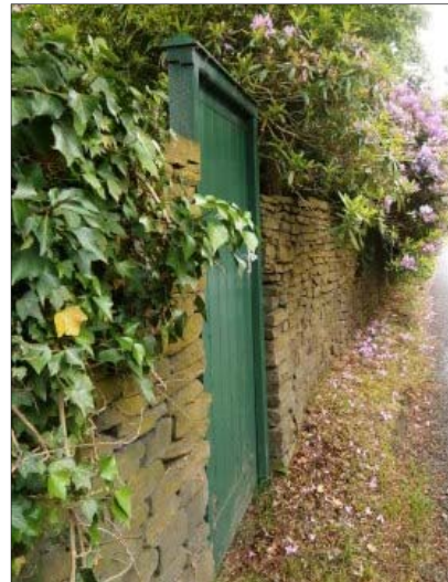
P6.16 Boarded door into the grounds of Pott Hall.
